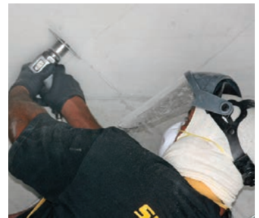
A Conco Spray Solutions crew member cuts grooves into the cleaned and prepped surface before applying the polyurethane coating material to ensure optimum adhesion and uniform coverage.
